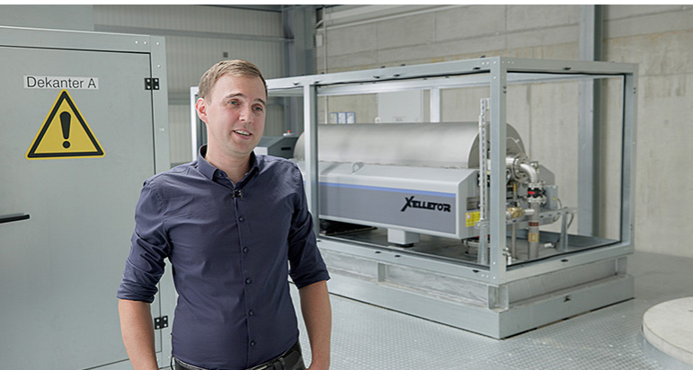
Wastewater master Manuel Ritter coordinated the modernization measures at wastewater treatment plant in Weinheim.
